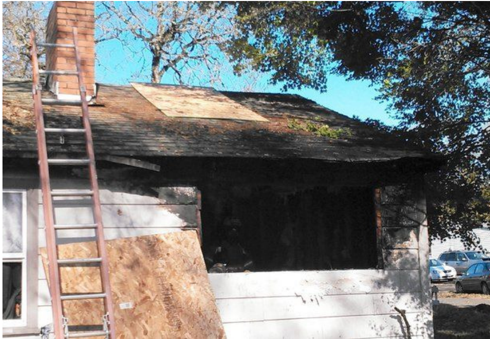
Fire broke out in a front bedroom of a Gladstone home, quickly spreading. (Gladstone Fire Department)
